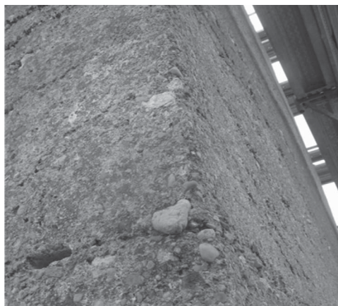
Figure 2. Corner of the tower that shows the continuity of the rammed earth wall (Vegas & Mileto).
