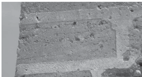
Figure 5. Strips of lime mortar sealing the joints at the top and the bottom of the tower (Vegas & Mileto).
